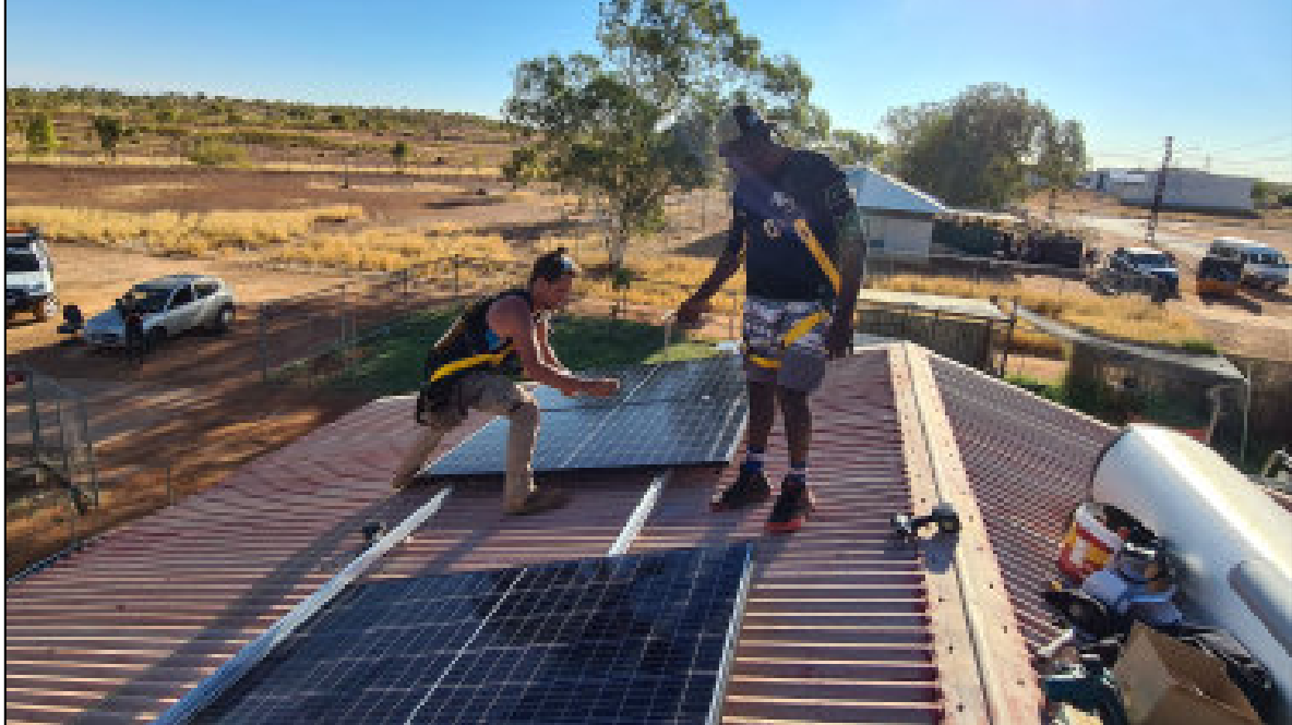
Andrew Dodd (right) learns the ropes on solar installation from Ben Hill at Tennant Creek.
