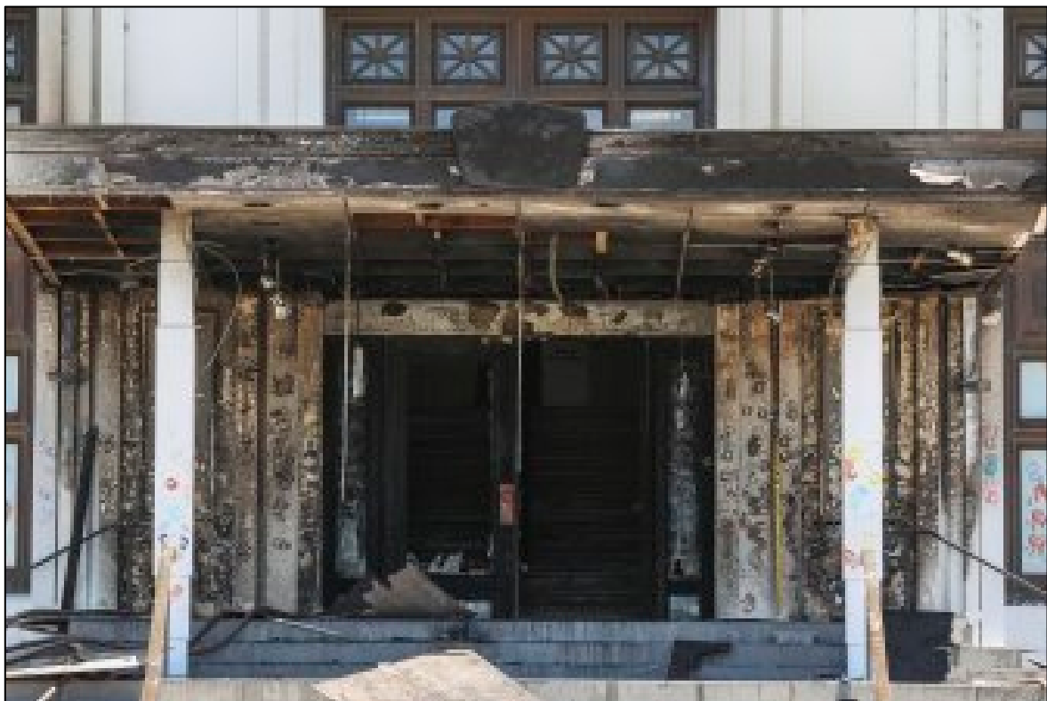
The fire-damaged front entrance of Old Parliament House.
